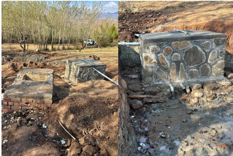
The picture above illustrates ongoing construction of a water source in Tebellong, Qacha's Nek, Lesotho
